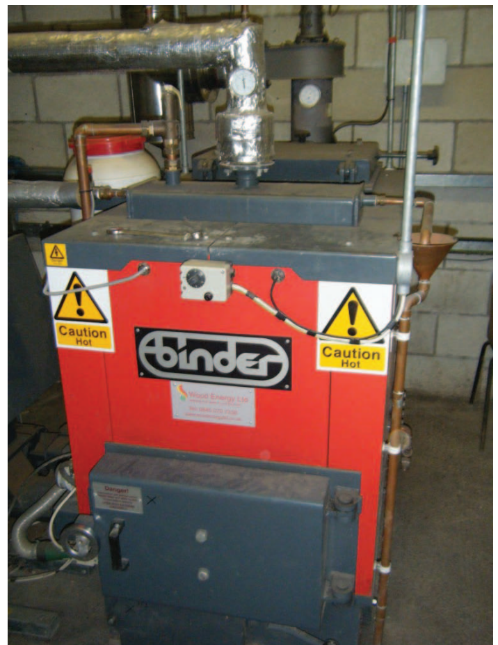
Woodchip Boiler Losehill
