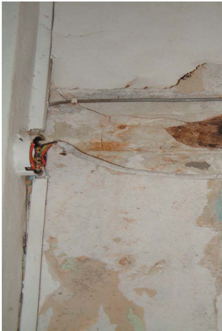
Results of water ingress - Photo: Alan Simons
