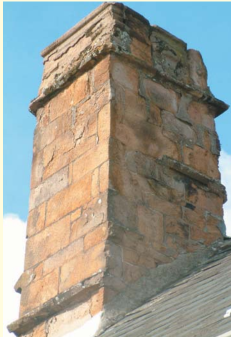
An unused chimney with no capping provision – Photo: Mark Clitherow
