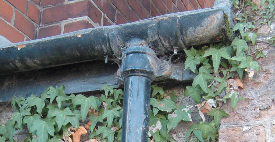
Check all guttering for effectiveness whilst it is raining - Photo: Alan Simons
