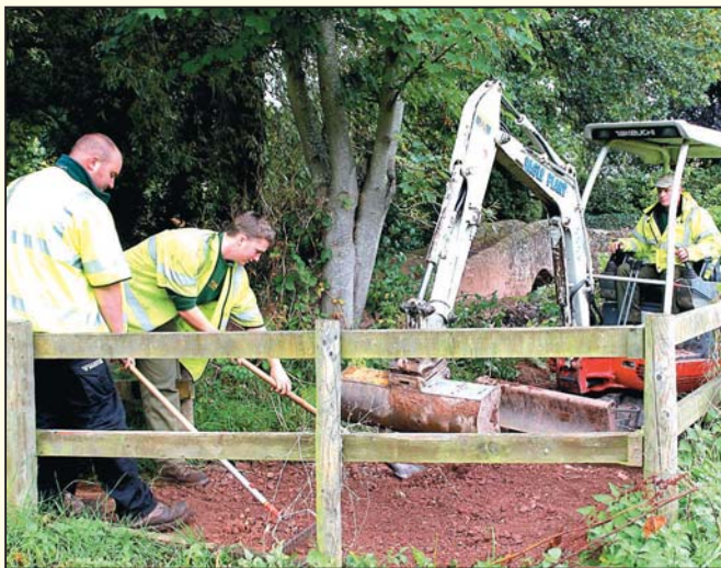
Rick Farmer (left), Tom Bird and Simon Lazarus (in the digger) from the field services team re-grading the path at Gallox Bridge in Dunster
